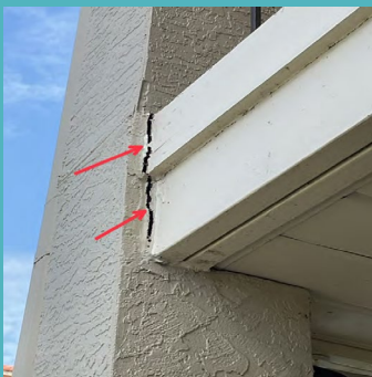
Building in Osceola County With Adhesion Failure of Sealant on Walkway
